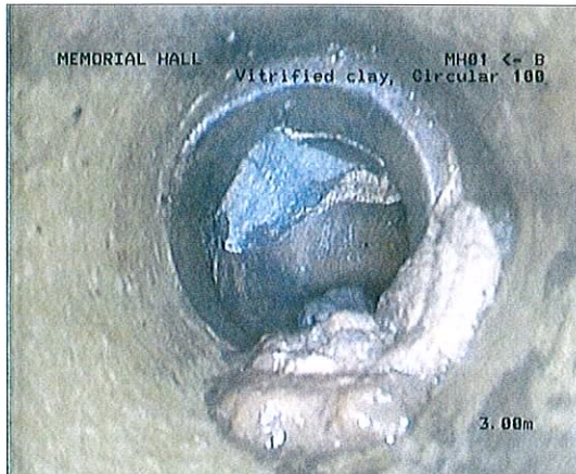
Photo: A_26_07_2013_16_6a.jpg, 00:00:00 3m, Encrustation medium at joint, from 03 to 07 o'clock, 15% cross-sectional area loss
