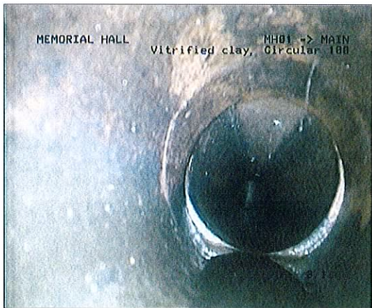
Photo: A_26_07_2013_29_6a.jpg, 00:00:00 8.18m, Circumferential Fracture at joint, from 08 to 02 o'clock
