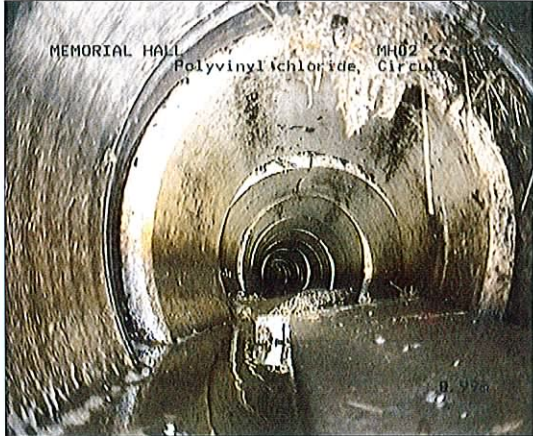
Photo: A_26_07_2013_40_4a.jpg, 00:00:00 0m, Obstruction, 20 % height/diameter loss Remarks: TIMBER
