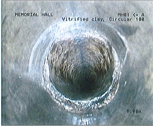
Photo: A_26_07_2013_5_5a.jpg, 00:00:00 1.98m, Circumferential Fracture at joint, from 09 to 03 o'clock
