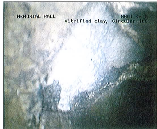
Photo: A_26_07_2013_18_8a.jpg, 00:00:00 3.24m, Hole in sewer from 08 to 11 o'clock
