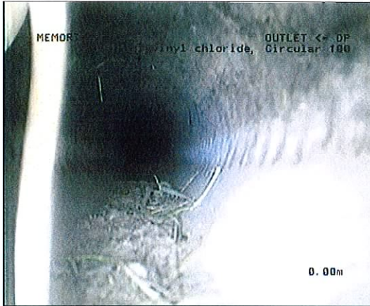
Photo: 6_1_4_08082013_161804_A.jpg, 00:00:00 0m, Debris, 10 % cross-sectional area loss, Start Remarks: PATCHY
