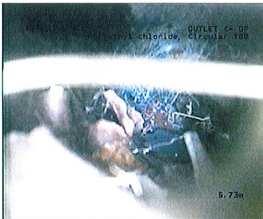
Photo: 6_1_10_08082013_161821_A.jpg, 00:00:00 5.73m, Debris, 20 % cross-sectional area loss
